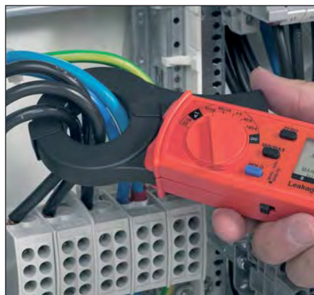
Differential current measurement with leakage current clamp
