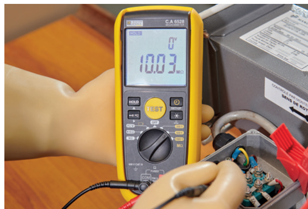
Preventive maintenance on a motor
