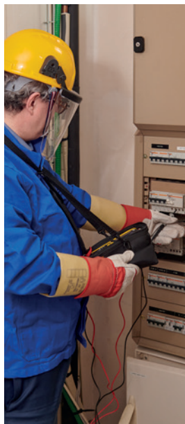
Control of an electrical cabinet
